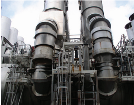
Aeropropulsion Systems Test Facility wind tunnel ducting and valves
